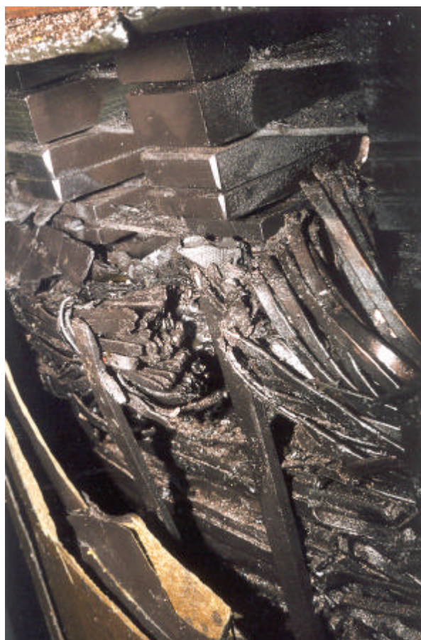
Fig. 3 November 1999 failure showing shorted turns and open strands involving Leg 2 of valve winding adjacent to top static ring
