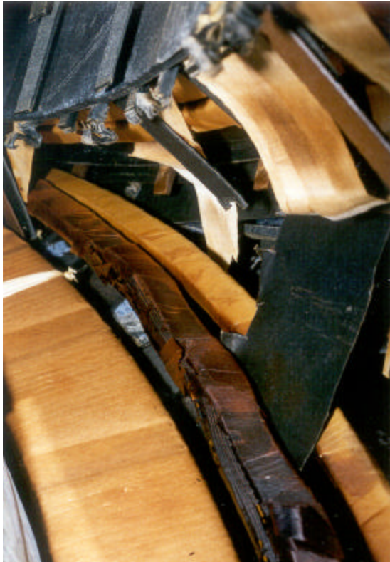
Fig. 4 February 2000 failure showing incinerated paper wrap on 1 of 2 CTC bundles of Leg 3 valve winding at top adjacent to static ring
