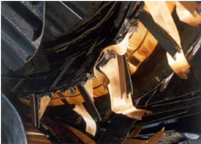
Fig. 6 February 2000 failure showing distorted CTC bundles of valve winding at top of Leg 2
