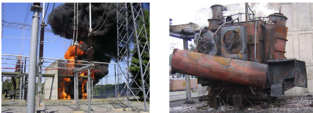
Figure 1 : Consequence of a bushing failure (735-kV transformer).
